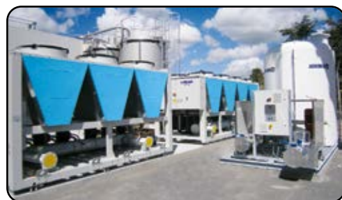
Chillers installed in France, * total cooling capacity 1155 kw
