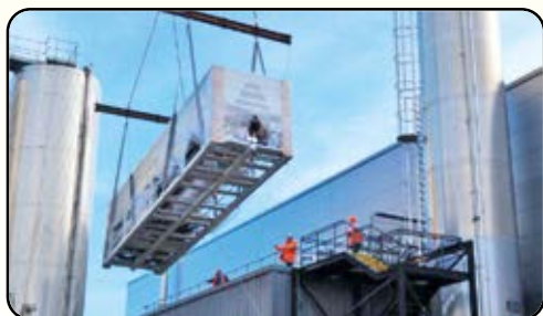
* Chiller installed in UK, 1070 kW
