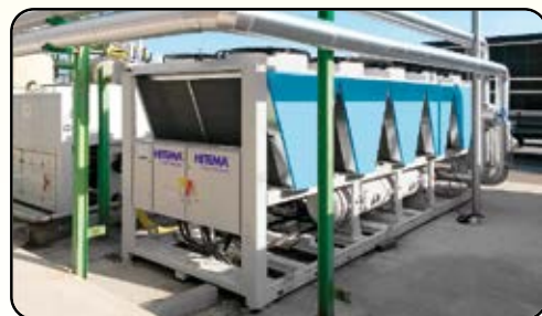
Chiller with Turbocor compressors, * installed in Spain, 780 kW
