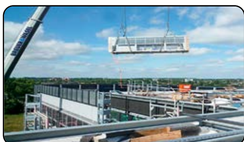
* Chiller installed in Dusseldorf, Germany, 820 kW
