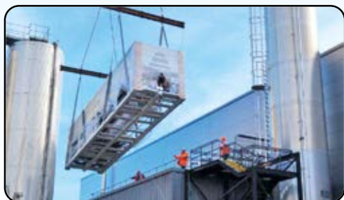
* Chiller installed in UK, 1070 kW
